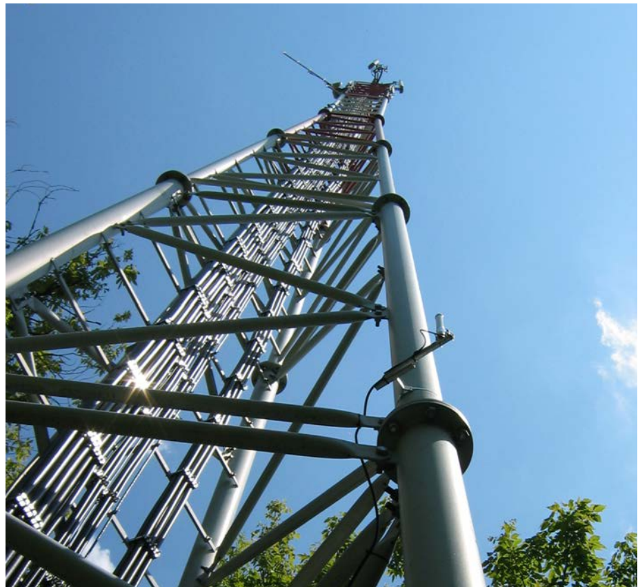
Inland AIS base station
